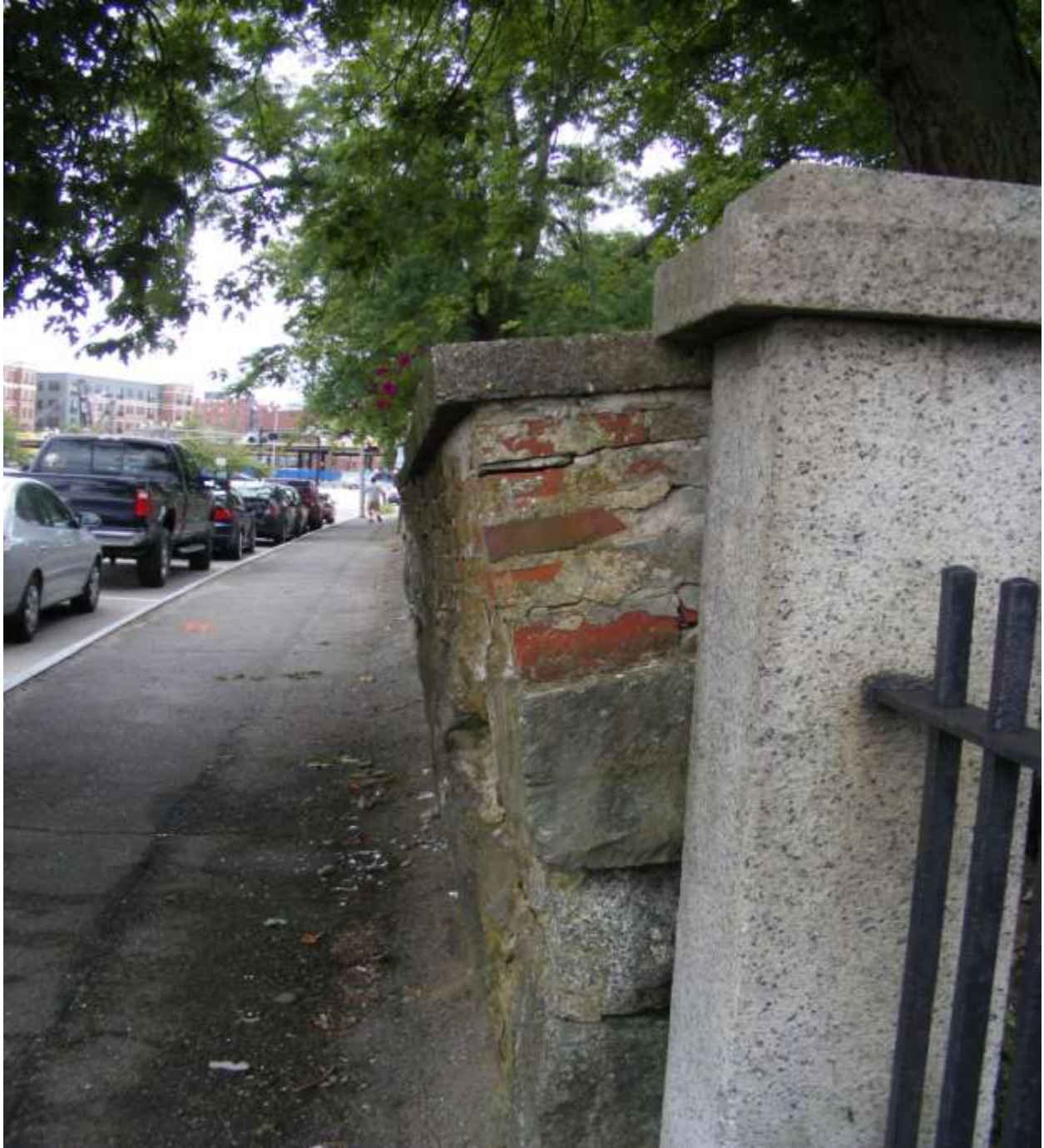
Cemetery Enclosure Fence and Stonework: Intersection between the North Cemetery and the Union Cemetery's enclosure walls.
